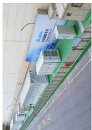
Delta Pingjhen Plant 5 MW / 3.6 MWh
