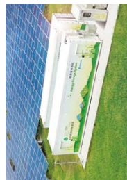
Kaohsiung Yong-an Solar Power Plant 1 MW / 1 MWh
