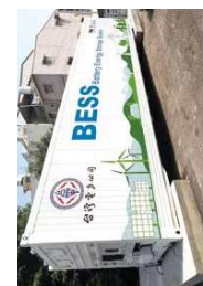
Taipower Fengshan Green Community 500 kW / 1 MWh
