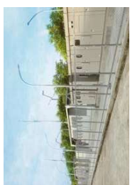
AIDC Taichung Factory 1 MW / 1 MWh
