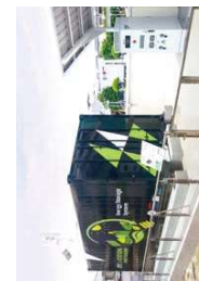
CPC Corporation Chaiji Gas Station 500 kW / 3 MWh
