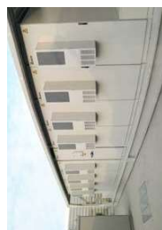
Changhua Coastal Park Solar Power Plant 1.5 MW / 1.5 MWh
